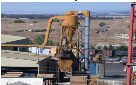
Cyclone at a Lumber Processing Facility
