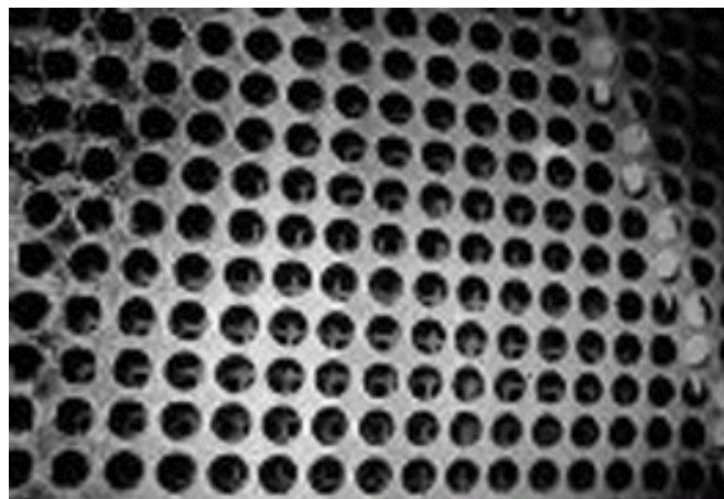
Figure 9-11. Gas distribution screens at the precipitator inlet
