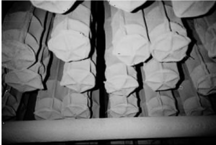
Figure 7-16. View of the bottoms of pulse jet bags
