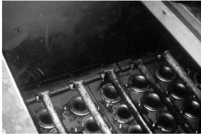
Figure 7-19. Compressed air delivery tubes
