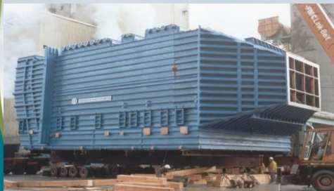
Record-size cross flow scrubber installed at B.C. kraft mill
