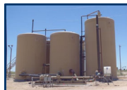
Typical Vertical Fixed Roof Tanks
