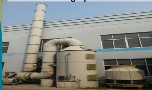
Counter-current Packed Tower at a Plating Operation
