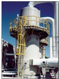
Packed Towers are primarily used for gas absorption.
