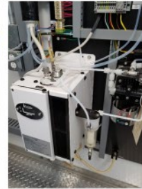
Extractive Conditioning System
