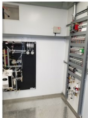
Inside a CEMS Shelter
