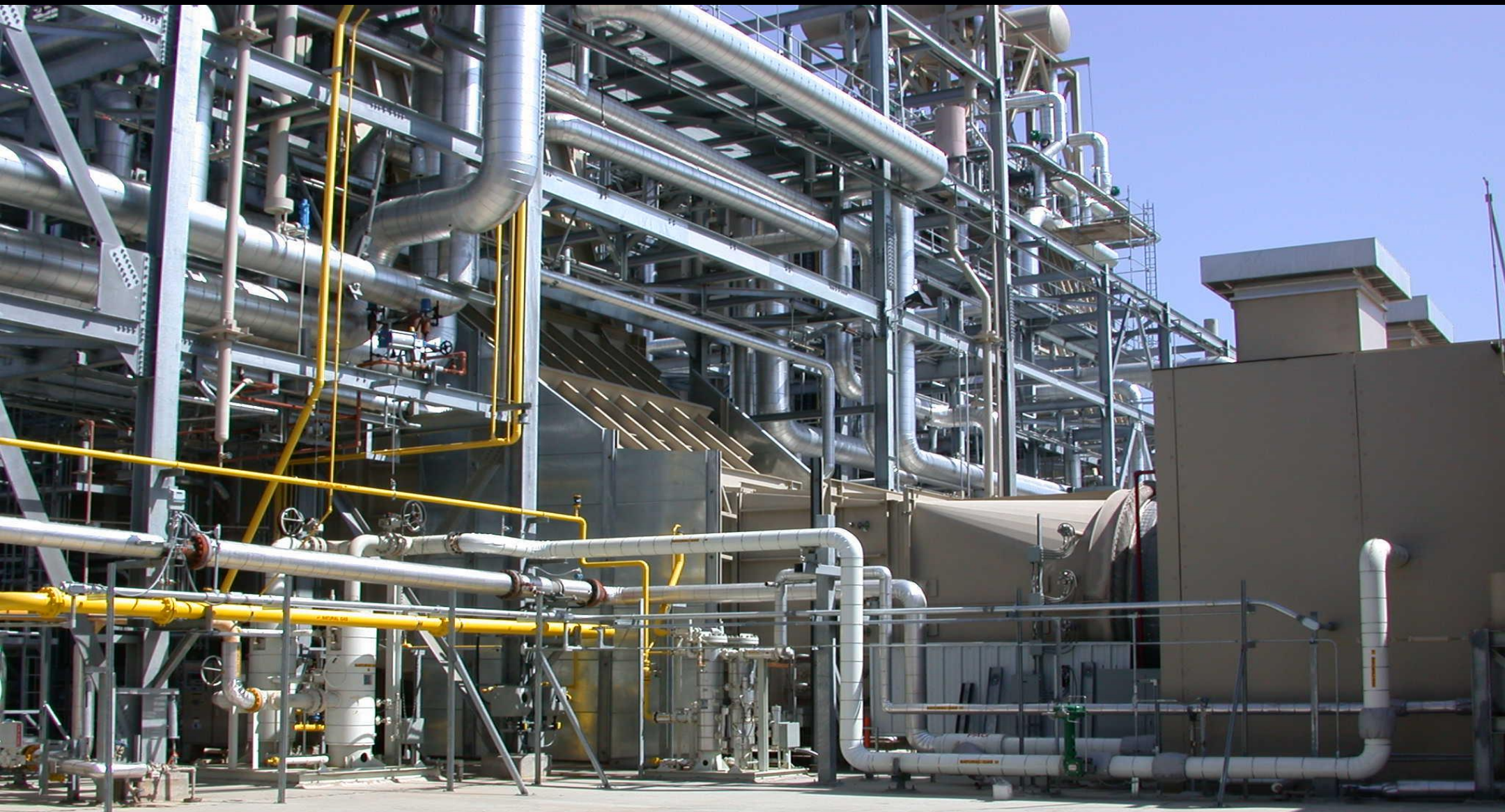
Steam Lines to Steam Turbine
