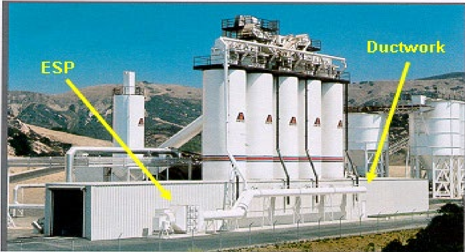
DUCTWORK TO ELECTROSTATIC PRECIPITATOR
