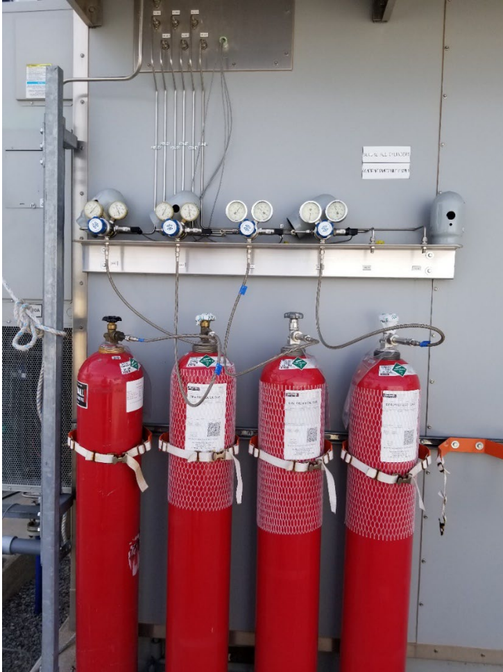
Cylinders of EPA Certified Gases
