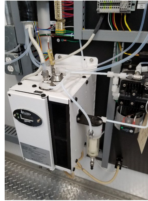
Extractive Conditioning System
