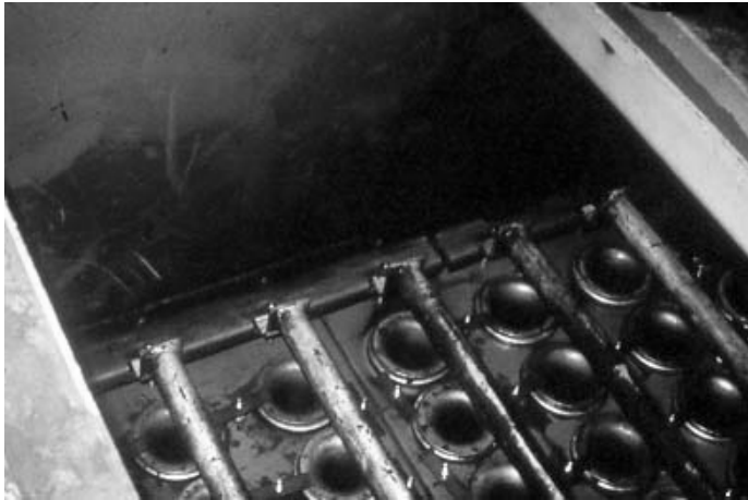
Figure 7-19. Compressed air delivery tubes
